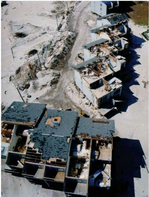
Plate 46 Property damage caused by Hurricane Fran.
